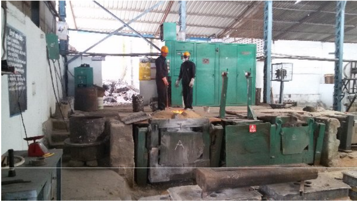
INDUCTION FURNACE - 450KW WITH THREE CRUCIBLE OF 1TON, 0.5TON AND 0.15TON
